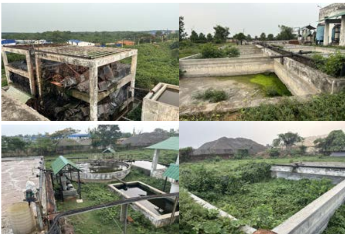
Figure-2: Photographs of CETP including Damaged Bio-Towers
