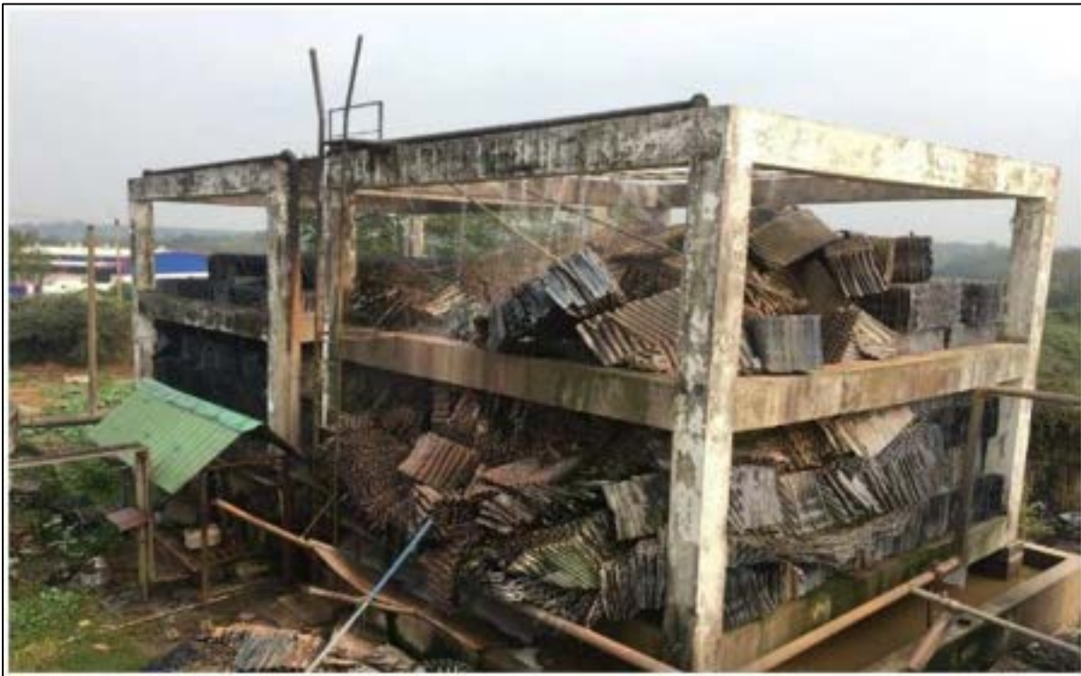
Figure 3-10: Present Condition of Bio-towers in CETP
